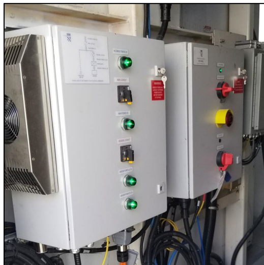
Figure 2: MineSense Edge Controller; Installed inside of shovel house
